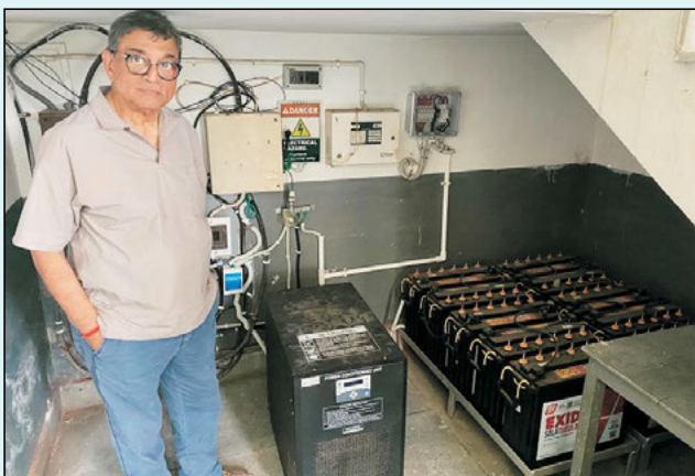
PP Rtn Tapan Rao visiting Solar Plant room partly funded by RC Singapore
